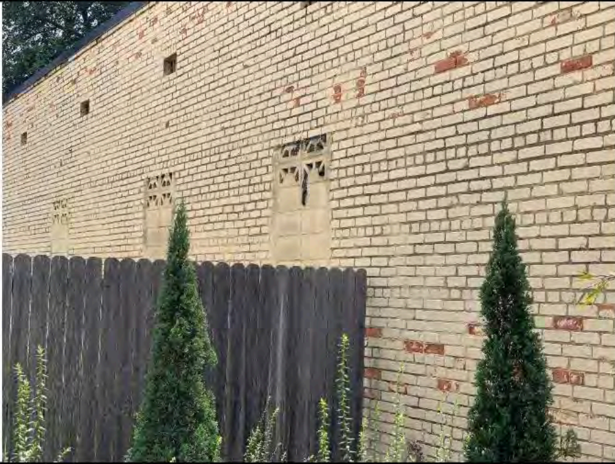
Photo 3: Partial eastern elevation – similar across entire elevation. Located along property line possibly.
