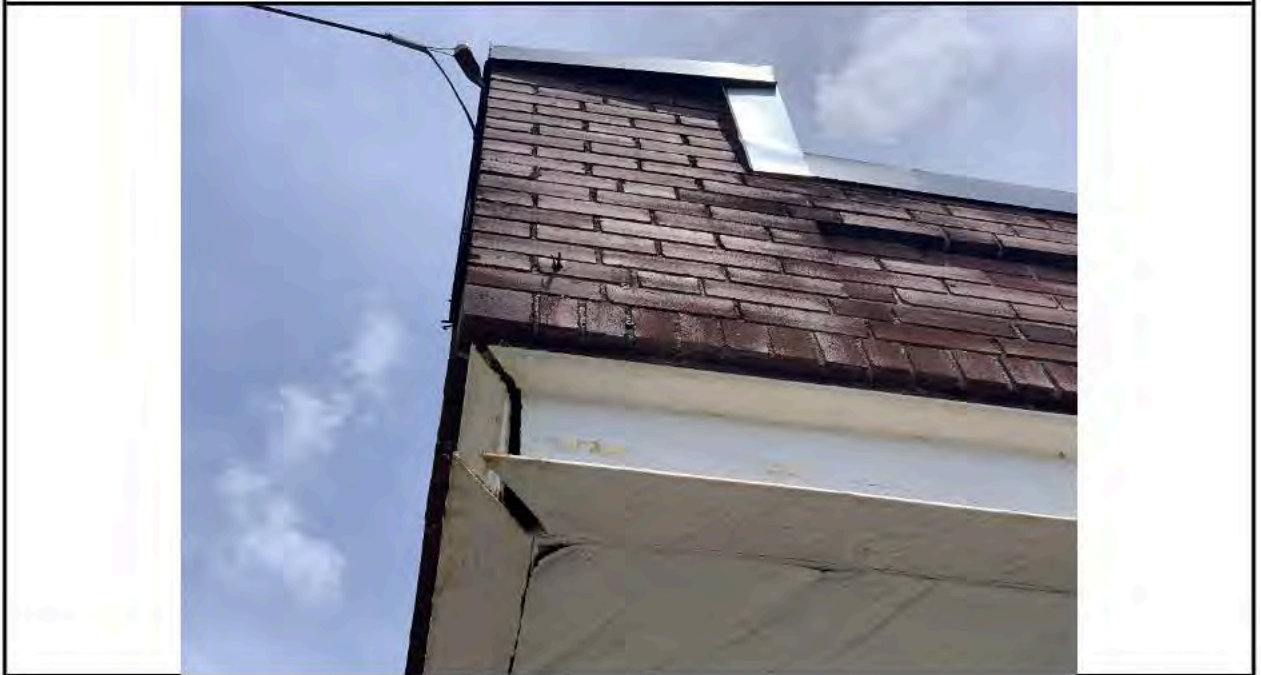
Photo 12: Northwest corner steel lintel with a gap in the connection over entry doorway.
