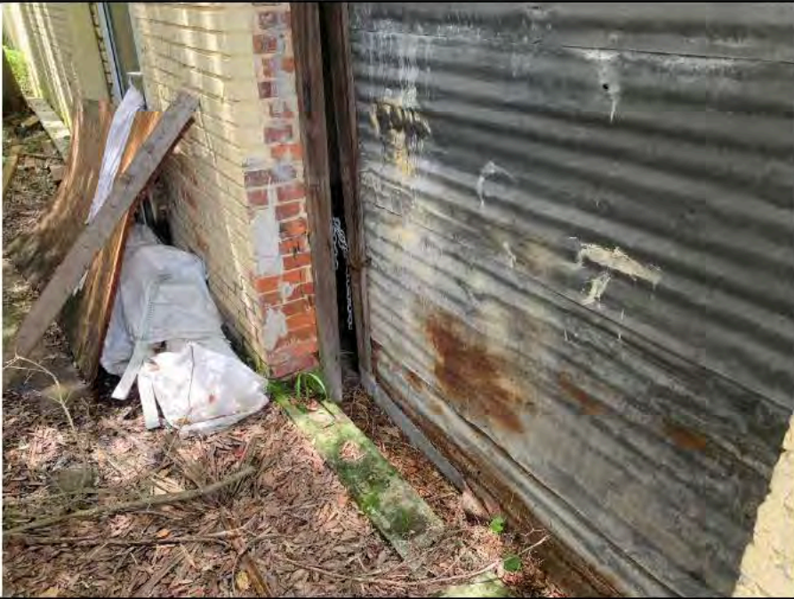
Photo 9: Southeast entry doorway which the sill is lower than the surrounding sidewalk allowing for direct water entry into the building.
