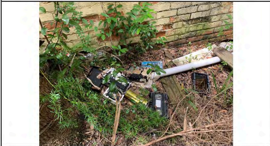
Photo 6: Damaged/missing brick masonry along south elevation.
