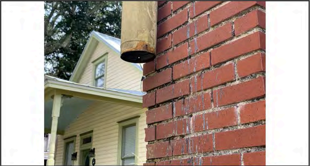
Photo 11: Section of missing downspout and mortar which is missing.
