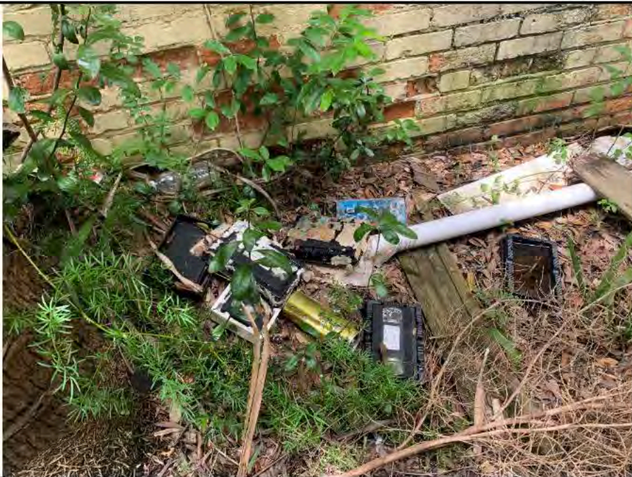
Photo 6: Damaged/missing brick masonry along south elevation.
