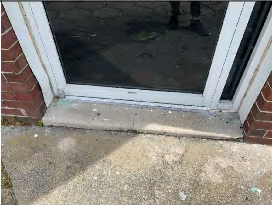
Photo 13: Typical thresholds with steps which do not meet ADA access requirements.
