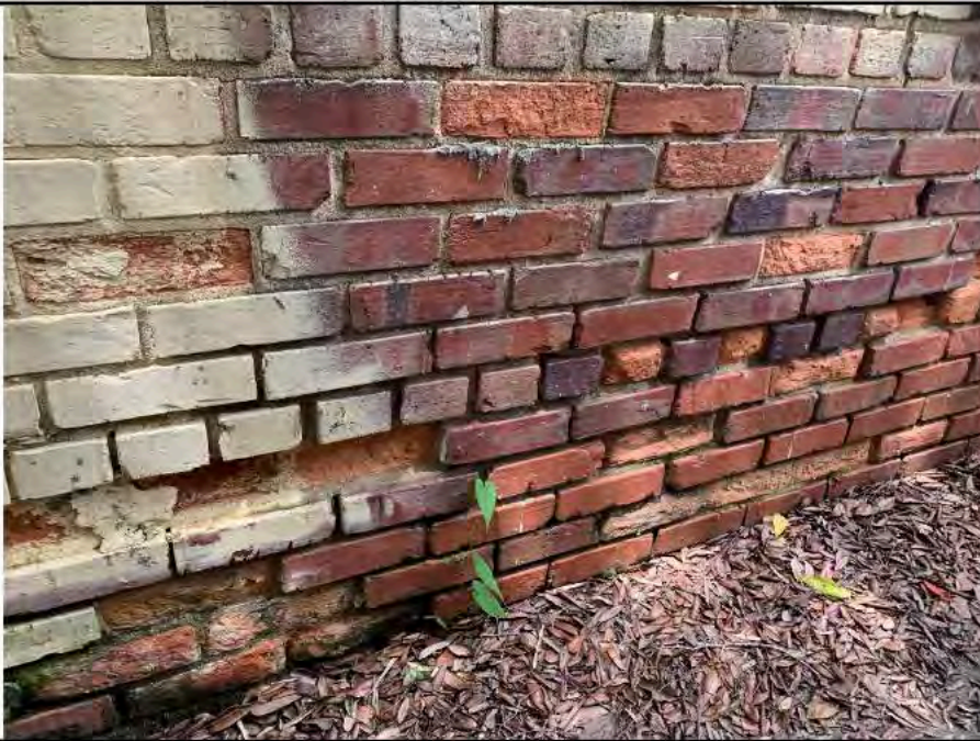
Photo 7: Damaged/missing brick masonry along south elevation.
