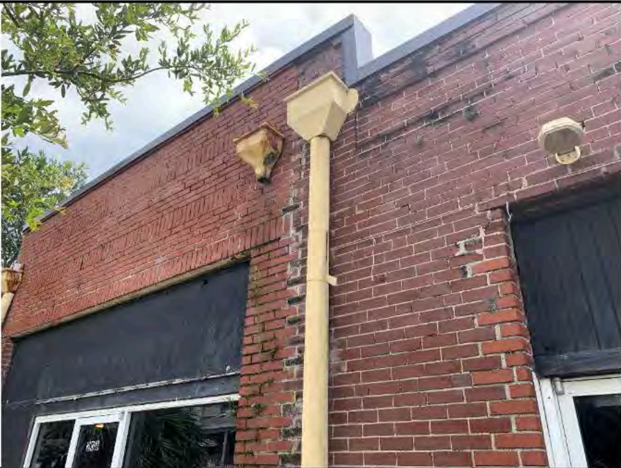
Photo 14: Current downspouts. Note poor brick mortar and heavy dirt.
