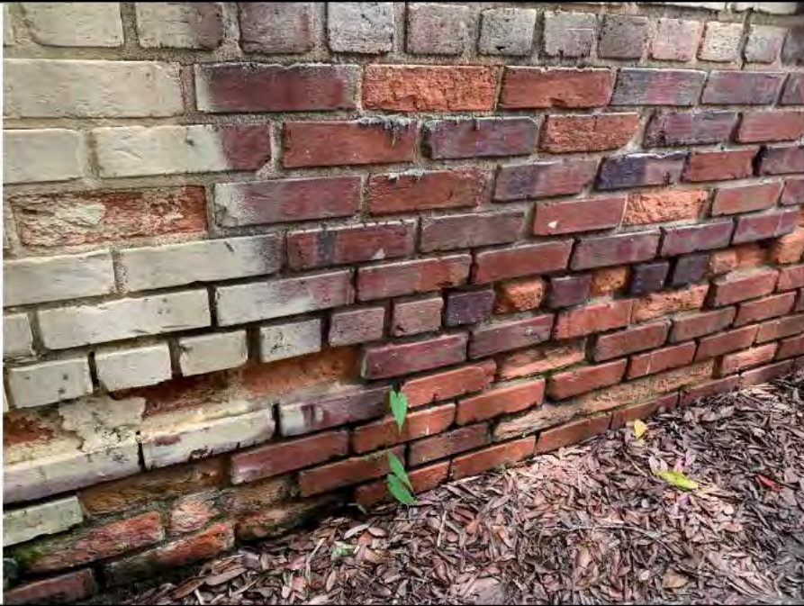
Photo 7: Damaged/missing brick masonry along south elevation.
