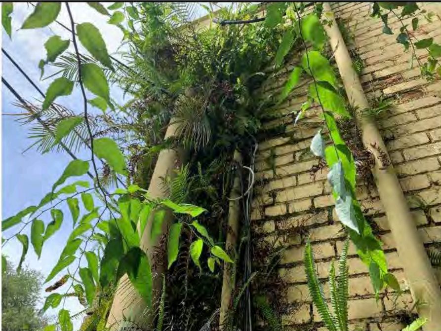
Photo 8: Heavy vegetation on southwest corner of the building. This corner has water intrusion likely from mortar damage.
