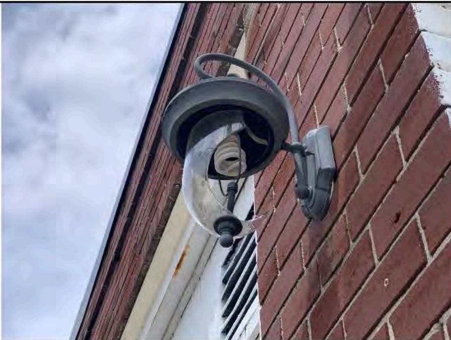
Photo 10: Broke globe at light fixture.
