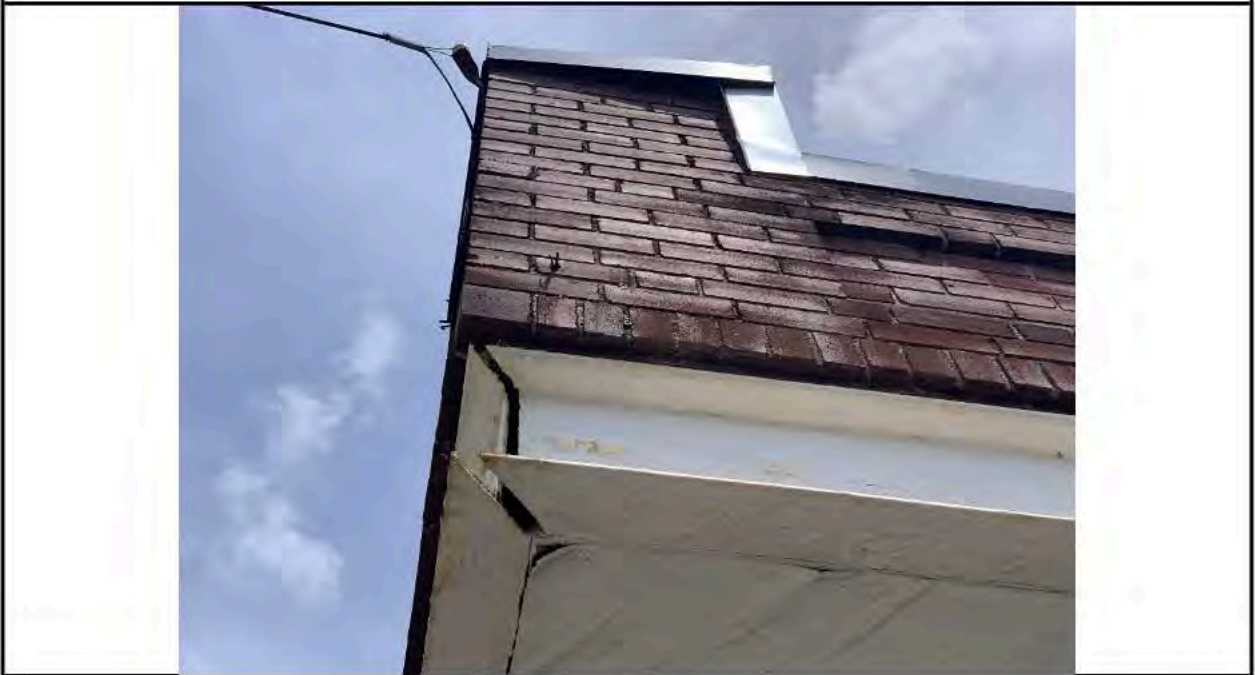
Photo 12: Northwest corner steel lintel with a gap in the connection over entry doorway.
