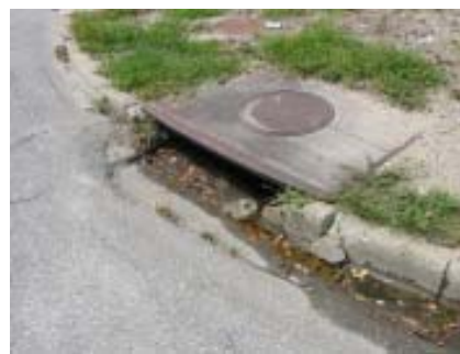
Aged and decaying storm sewer inlet on Stockton Street
